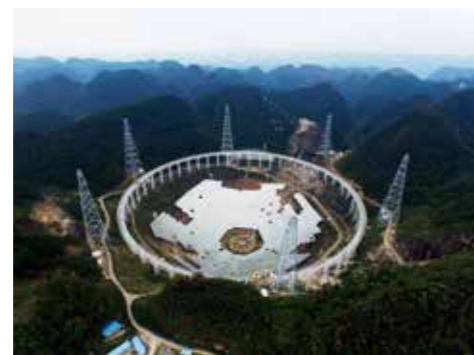
索网结构及反射面单元安装 Cable-net structure and installation of reflector units
